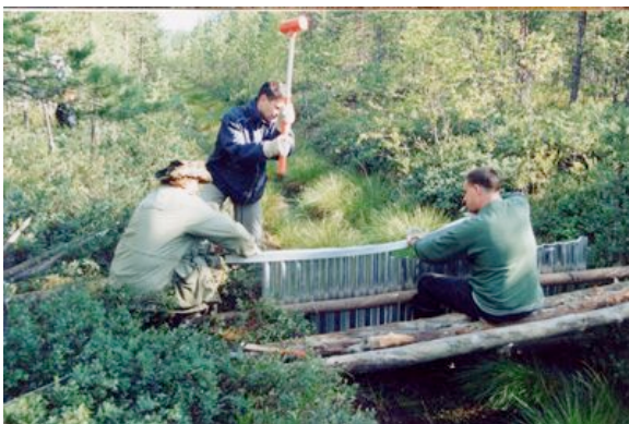
Repairing drainage in a Russian peatland during a PBP follow-up project. Photograph: Alexander Mischenko.
